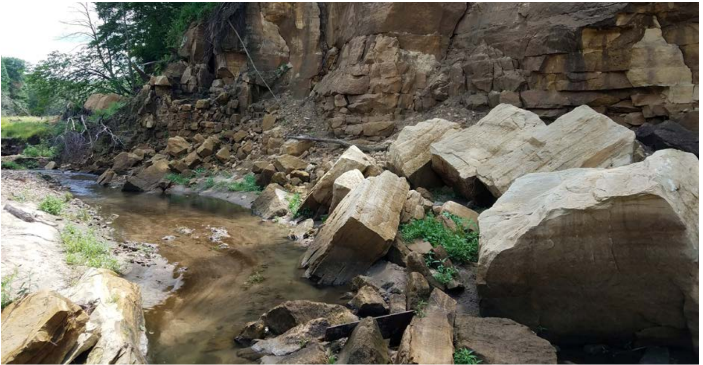
One of the breached dam sites in the Coon Creek Watershed. Photo by Eric Booth
