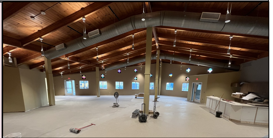
Above: A look inside the Life Center during construction. This larger space will be used primarily for the YWCA childcare program.
